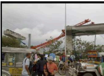
Skyway 2 crane ruin in SLEX Skyway crane collapsed along SLEX and Bicutan Ext. Louie Fababser | 2010-07-14 | Parañaque City Metro Manila 150
