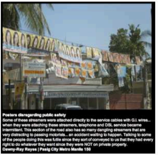
Posters disregarding public safety. Some of these streamers were attached directly to the service cables with GL wires... when they were attached these streamers, telephones and DLS service become intermittent. This section of the road also has so many dangung streamers that are very distracting to passing motorists... an accident waiting to happen. Telling to some of the people doing this was futile since they sort of conveyed to us that they had every right to do whatever they want since they were NOT on private property. Dewey-Ray Reyes | Pasig City Metro Manila 150
