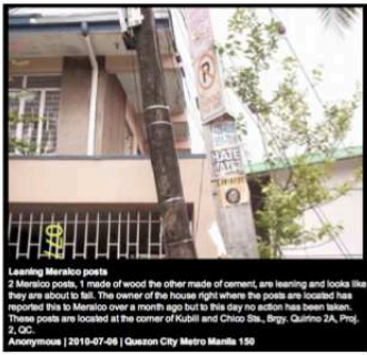
Leaning Merlito posts 2 Merlito posts, 1 made of wood the other made of cement, are leaning and looks like they are about to fall. The owner of the house right where the posts are located has reported this to Merlito over a month ago but to this day they still have been fallen. These posts are located at the corner of Kubli and Chico Sts., Brgy. Quirino-2A, Phil., 2, QC. Anonymous | 2010-07-08 | Quezon City Metro Manila 150
